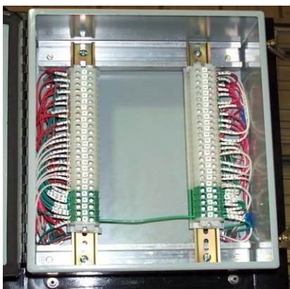
Control Panel pre-wired and tested
