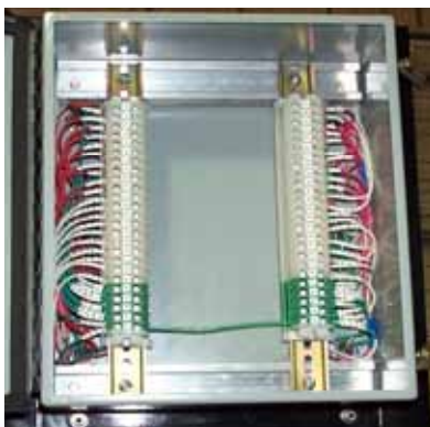
Control Panel pre-wired and tested
